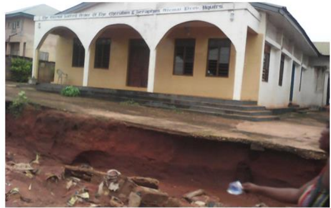
Plate 4: Picture showing the dilapidated building at Abu Inumoru street, Aibotse.
