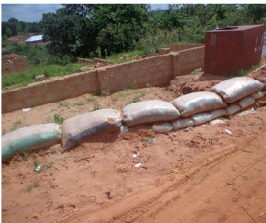
Plate 5: Shows a site at Iyekhei, Auchi where sand bags are used to control erosion
