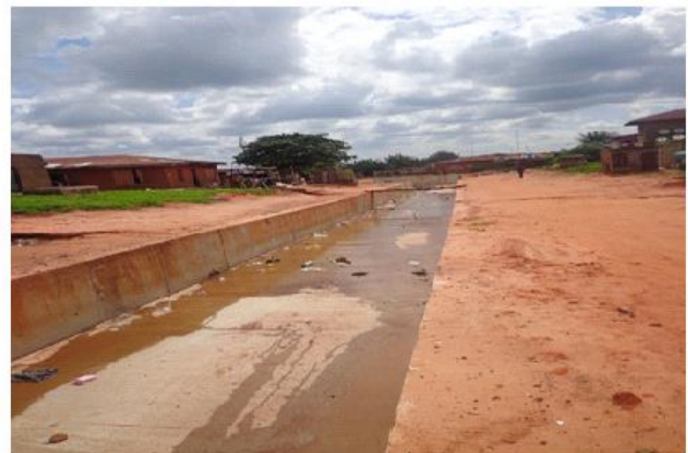
Plate 6: Shows a drainage constructed by SETRACO Company at back of Union Bank Usogun.
