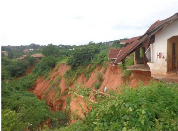
Plate 1: Shows a house affected by the gully erosion at Old Zongo area, Usogun, Auchi.
