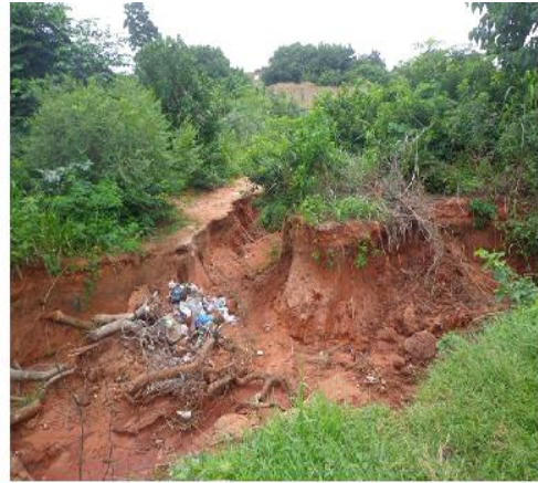
Plate 2: Shows an erosion site at chairman street Iyekhei, Auchi.
