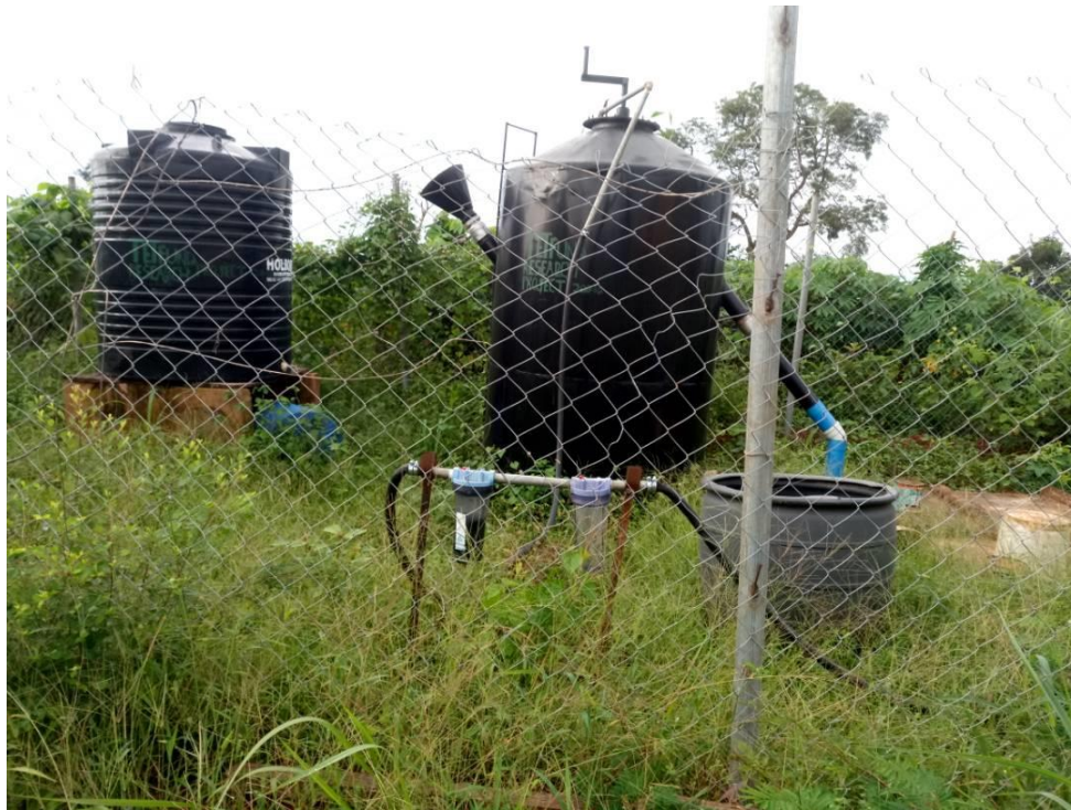
Figure 2 Installation and Experimentation site of the Bio-digester in Auchi Polytechnic Demonstration farm
