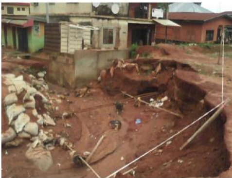
Plate 3: Picture showing a road affected by gully erosion at Aibotse.
