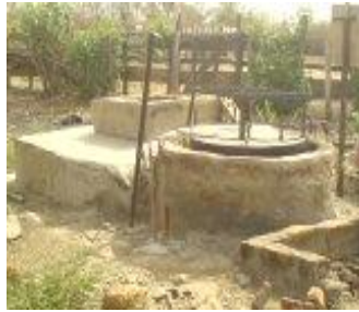
(a) Biogas plant
